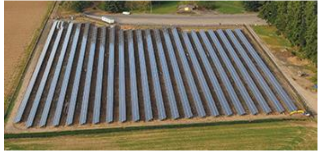
Oregon DOT-installed 1.75 MW solar array at the French Prairie Rest Area on I-5
