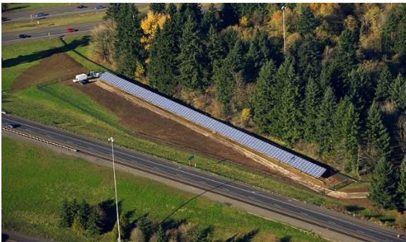
Oregon DOT-installed solar array at the interchange of I-5 and I-205 near Portland
