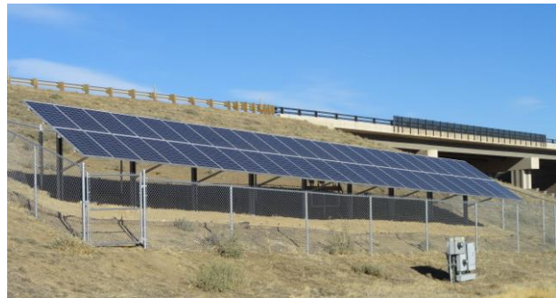
Solar panels along Northwest Parkway near Denver, Colorado
